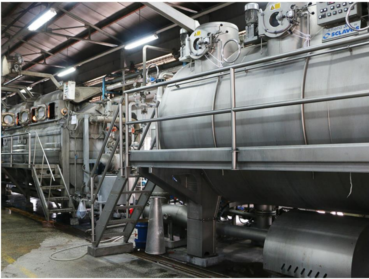
Picture-3: Inside View of the Fabric Dyeing unit.
